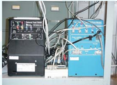
Data Acquisition / Control Devices
